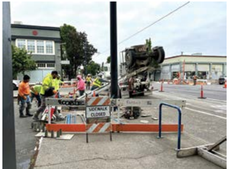
Contractors working for PBOT pour a new ADA ramp corner at SE Salmon St. and Grand Ave. Photo by PBOT.
