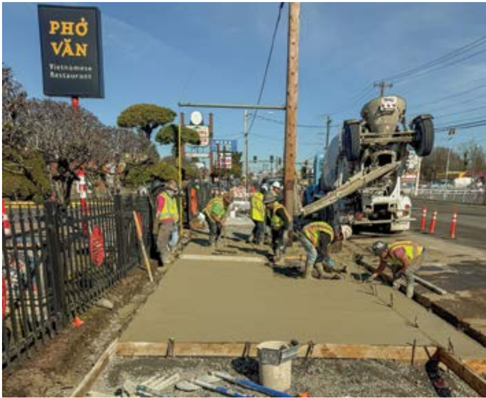
Construction along 82nd Ave. in 2025. Similar efforts will continue in 2026. Photo by PBOT.
